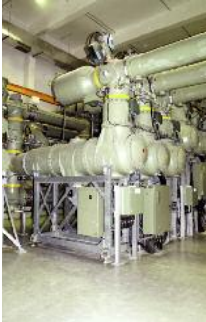
GIS circuit breakers
