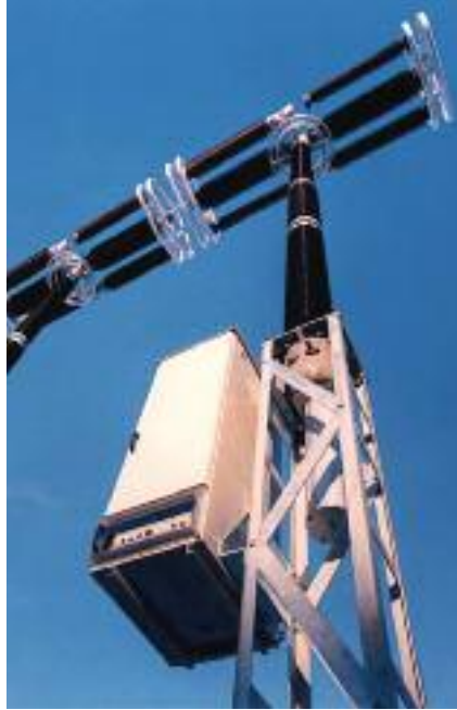
Live tank switchgear
